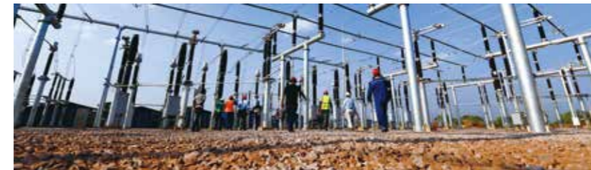
▲ Lualaba Copper Smelter and the DRC State Grid Corporation jointly build the southern Kolwezi Converter Station.
